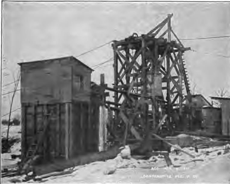
PLATE 82a.—Contract 12. Headframe and Measuring-box at Shaft 4. Water from tunnel was measured by orifice, the head on which was obtained by Friez Automatic Stage Recorder. Trans. Am. Soc. C. E., LXXIII, 1911.
